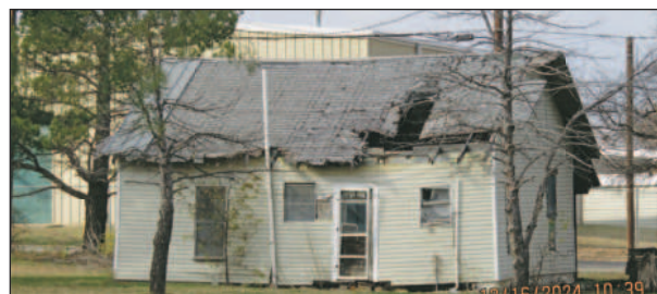
A property at 302 N. Graham that was deemed dangerous by the city of Breckenridge and was part of a discussion by the city commission.
