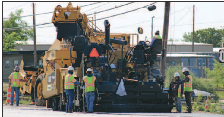
A change order was approved Tuesday, Jan. 7 for the city's Street Improvement Project - Phase 1. The change order includes seven modifications with to the contract with Raydon, Inc.
